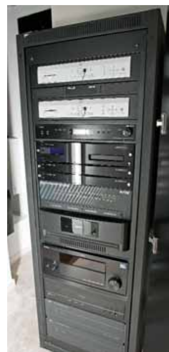
Crucial but intrusive technology is hidden safely out of sight
